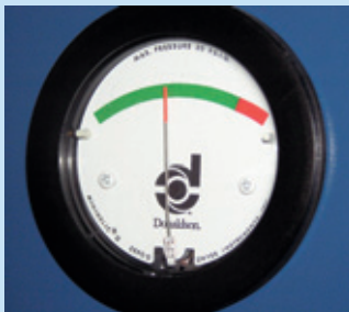
Differential pressure gauge(s) identifies filter maintenance
